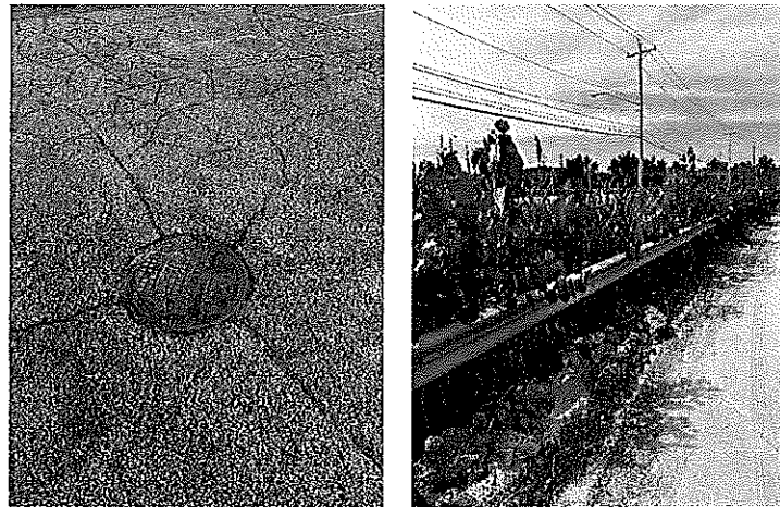
Figure 6: Cracked asphalt pavement; failing safety guardrail. McBride Dale Clarion site evaluation photos, Photos Captured: 24 July 2026.
