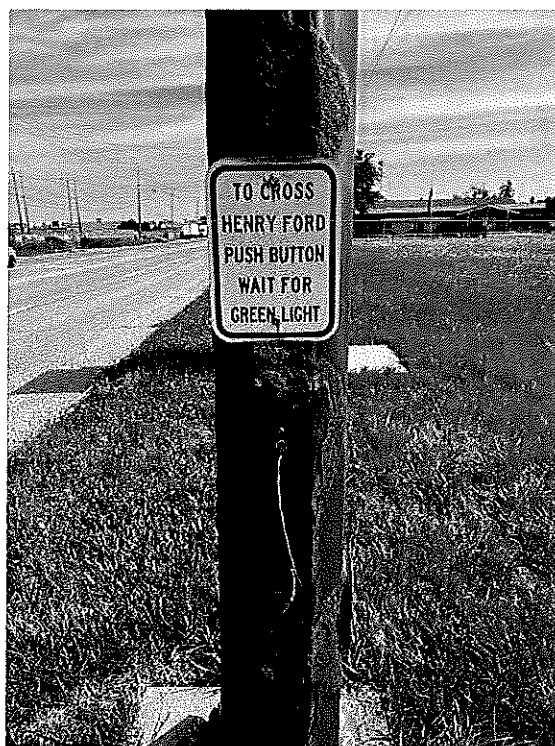
Figure 10: Off-site traffic light pole is rusted and deteriorating (located Northeast of intersection of Hummel Road and Engle Road). McBride Dale Clarion site evaluation photos, Photos Captured: 24 July 2026.
