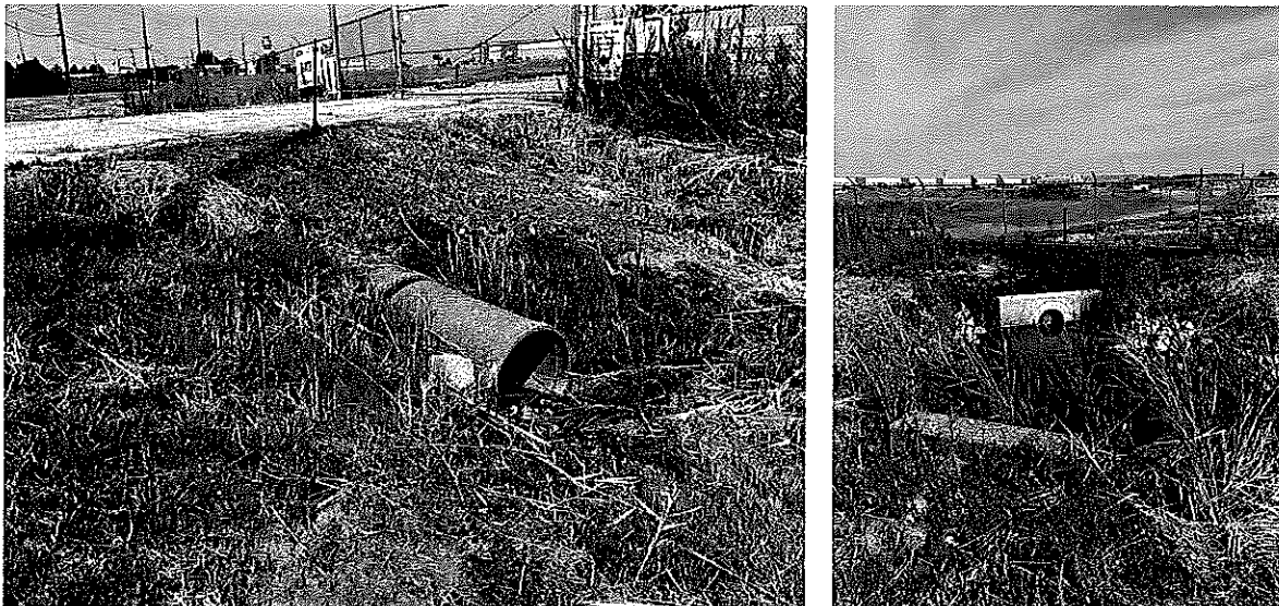
Figure 12: Off-site entrance culvert with standing water and broken sidewalk/sewer collection cover. McBride Dale Clarion site evaluation photos, Photos Captured: 24 July 2026.
